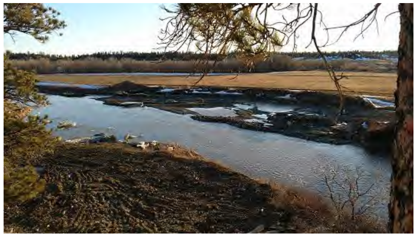
3/12/2017 Diversion removed flow back to main channel bench and willow lift work remaining
